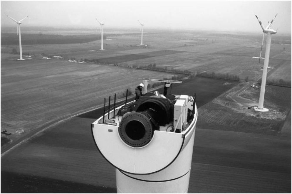
Figure 6.18 Turbine Assembly in the Air (1). (View of nacelle of 1.5 MW NEG Micon turbine after installation of low-speed shaft (front) and gearbox. The ring of bolt holes in the low-speed shaft flange for hub mountings are clearly visible). (Reproduced by permission of NEG Micon)
