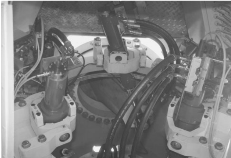
Figure 6.9 Blade Pitching System Using Separate Hydraulic Actuators for Each Blade. (Each actuator cylinder is supported on gimbal-type mountings bolted to the hub, and its piston applies a pitching torque to the blade via a cantilevered conical tube eccentric to the blade axis. The blade is attached to the outer ring of the pitch bearing).
